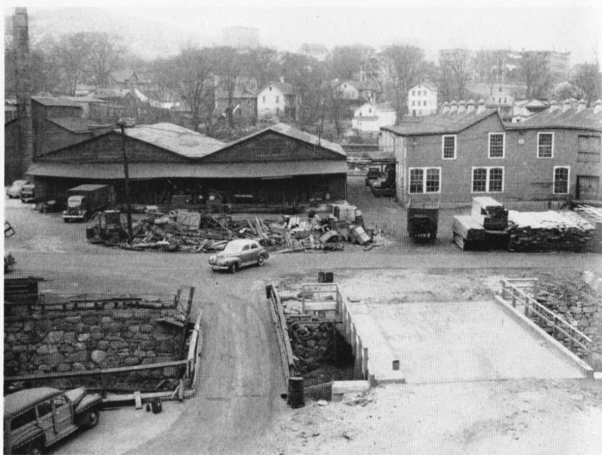
Here is a view of the old and new bridges which span the Mad River. The picture was snapped from Building 109-3 and shows the vast improvement of the new, wide bridge over that of the old, narrow one.
